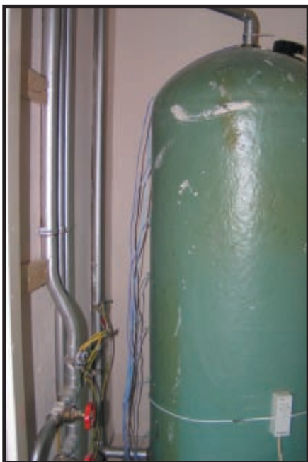
Photo 3—I waited until my wife was out before I "installed" the system as I thought cutting the foam might have been messy! Luckily, it was easy to bore out small plugs and mount the sensors against the copper cylinder.
